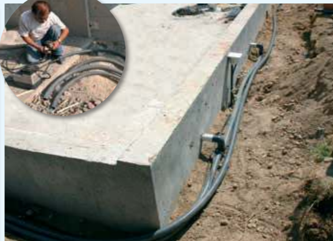
Installation and pressure testing of the pipe system for inlet fittings and skimmer.
