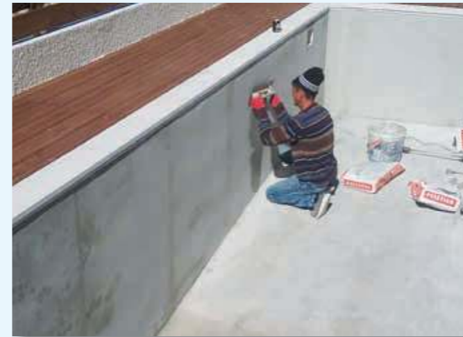
Super Plast coat is smoothly placed over the pool walls and bottom to make the surface smoother for more protection of the PVC Membrane.
