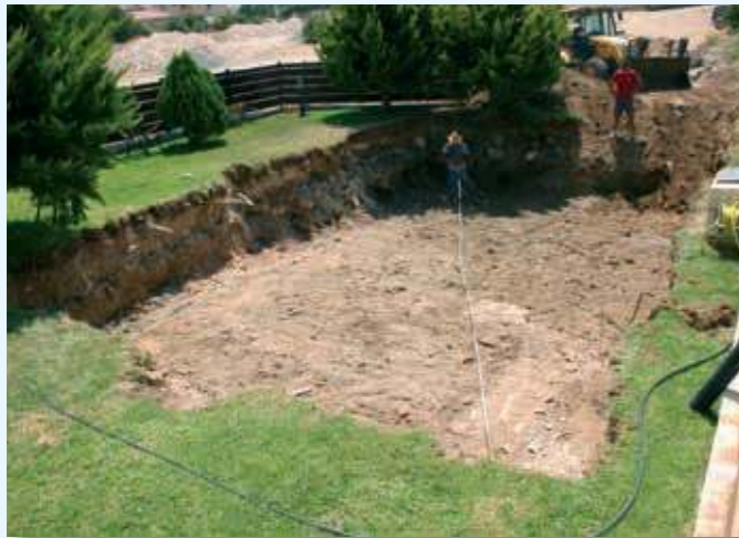
After chalking out the ideal location you have chosen for your pool, experienced excavators dig the proper depth and size of your particular design. Your yard begins its transformation!
