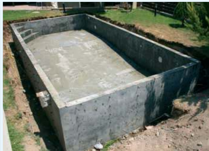
A smooth, full 20cm thick seamless reinforced concrete pool structure is formed to last for centuries.
