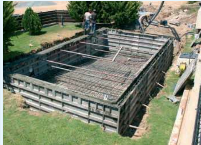
Iron reinforcement is placed and a full 20cm thick concrete wall is erected.
